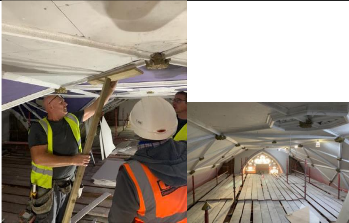
The ceiling in the main hall was also unstable, working with EAC and HES as well as specialists the design team were able to identify a method of retaining the existing details without fully renewing the ceiling, a solution that was acceptable to all.
