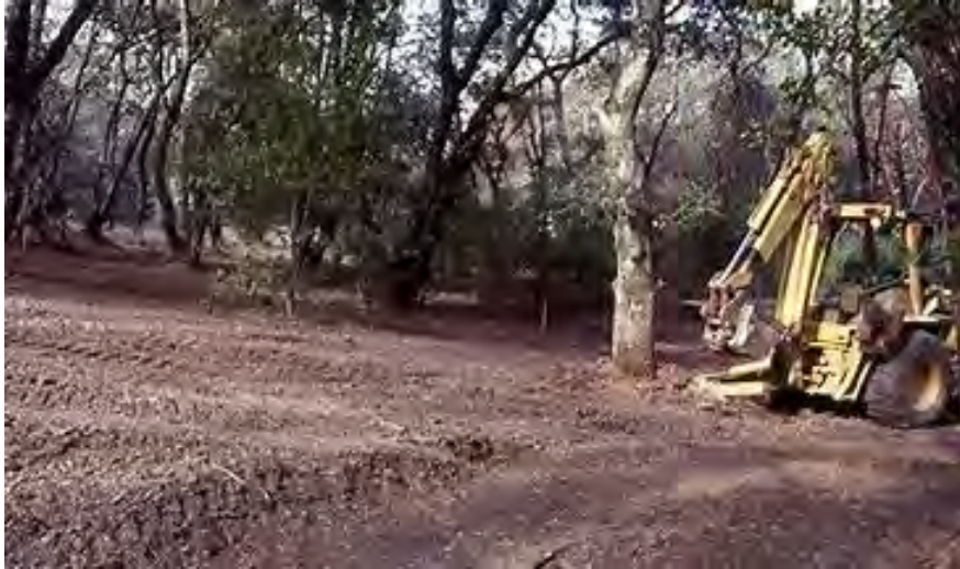
Construction: Compaction of tree roots from works being located too close to existing tree on site, with no Root Protection Zone set out in fencing.
