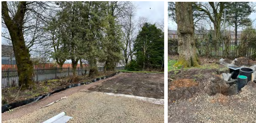
Construction: Tree roots severed by the development works (implementation of drainage).
