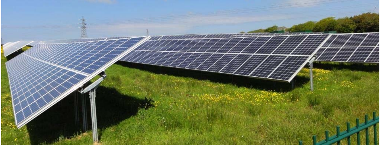
Figure 6: Free-standing solar arrays, The Renewable Energy Hub, https://www.renewableenergyhub.co.uk/
